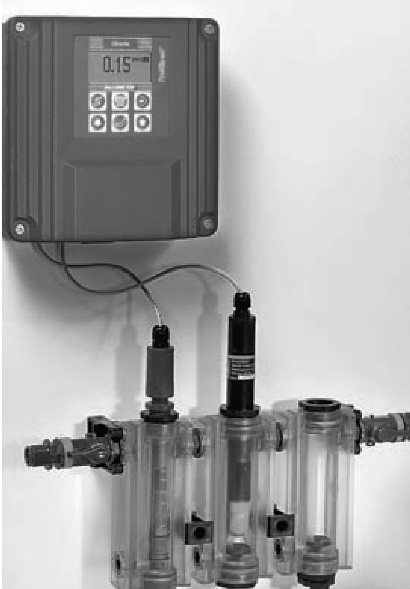
Fig. 1. Integrated BOD flow trough systema "Strix" plc., Zagreb, Croatia
